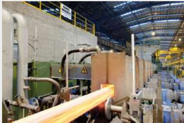
Fig. 11: Billet before reheating at the inlet of the Elotherm EloHeat™ system at Tung Ho Steel in Taiwan (source: SMS Elotherm)
